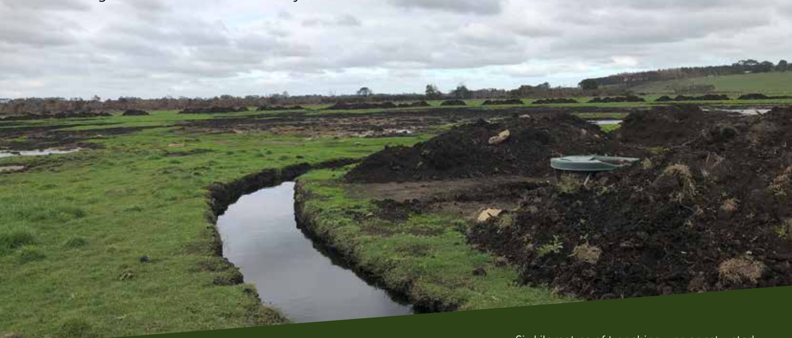
Six kilometres of trenching was constructed and filled with water, as the main fire control strategy at Cobrico.
